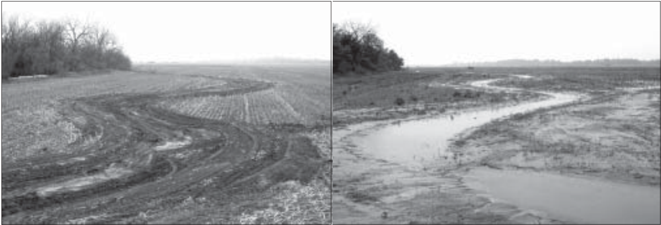
In lowland areas, such as the Platte River valley, excavating fill material can create a shallow water wetland that can be seeded to a marsh or wet-mesic prairie community.
