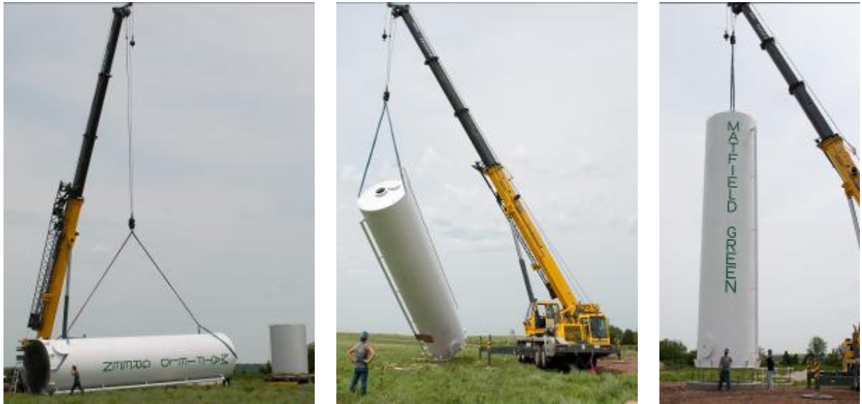
New water tank arises on the west side of Matfield Green. It officially went into service at 10:05 pm on Saturday, June 11, 2011. [Photos by Jim Worster]
