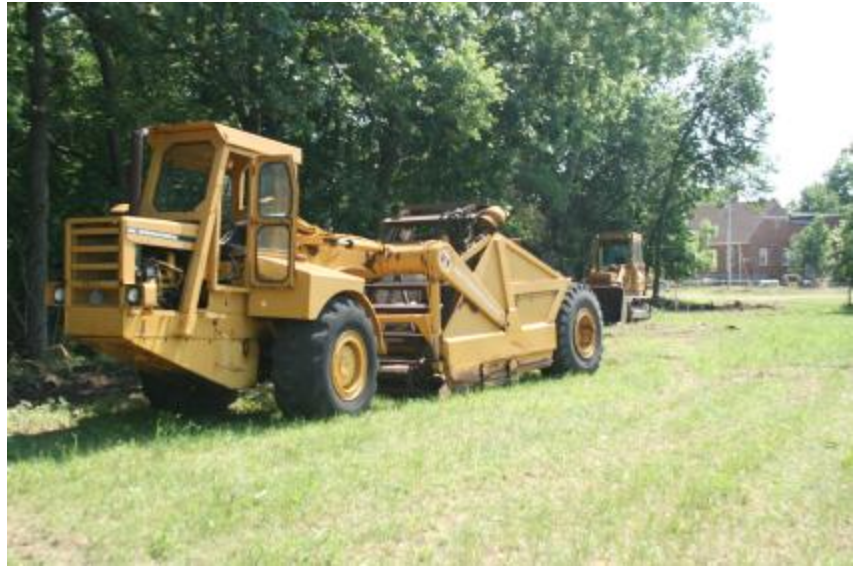
Heavy equipment in northeast Matfield Green signals the start of the fire station construction project.
